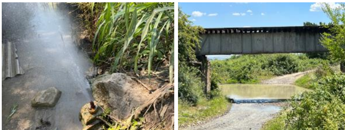
Figure 31: Leakages due to damaged system
