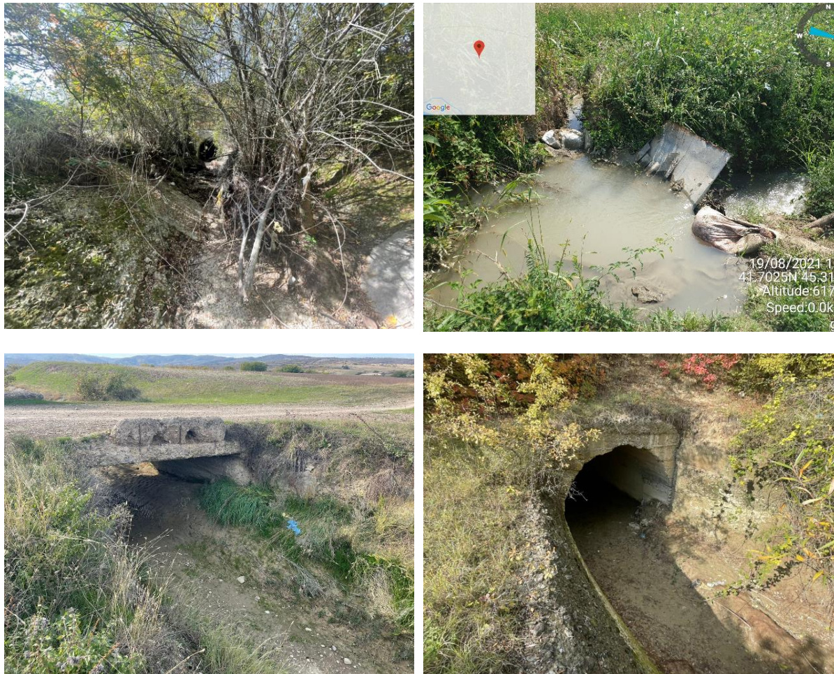
Figure 6: Condition of the Main Canal 15
