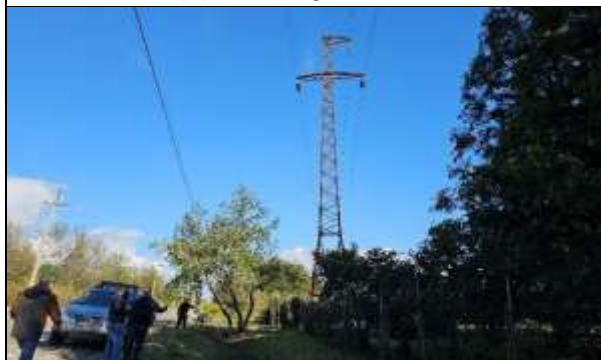
(c) Power-line Tower along the Rioni River
