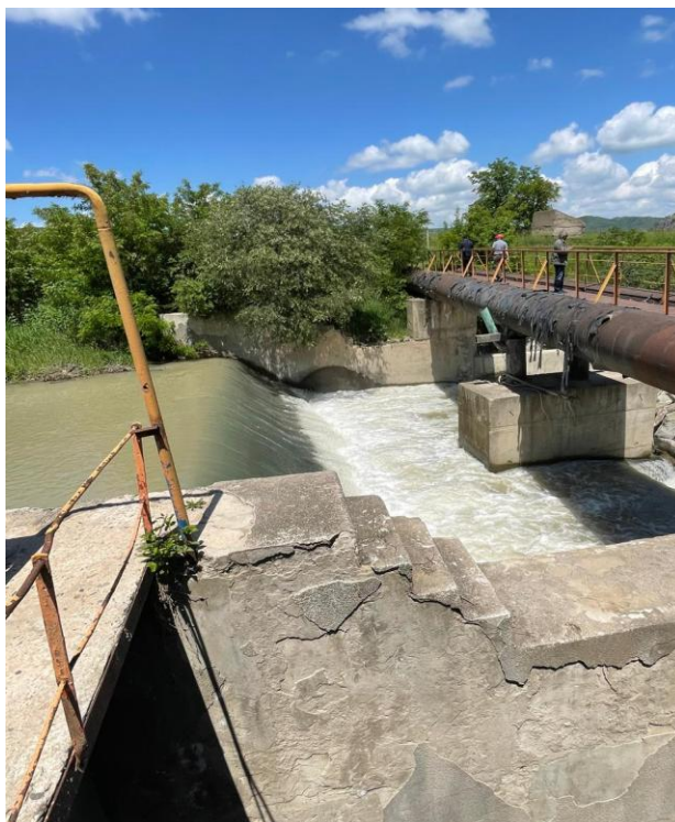
Headworks at Mashavera River
